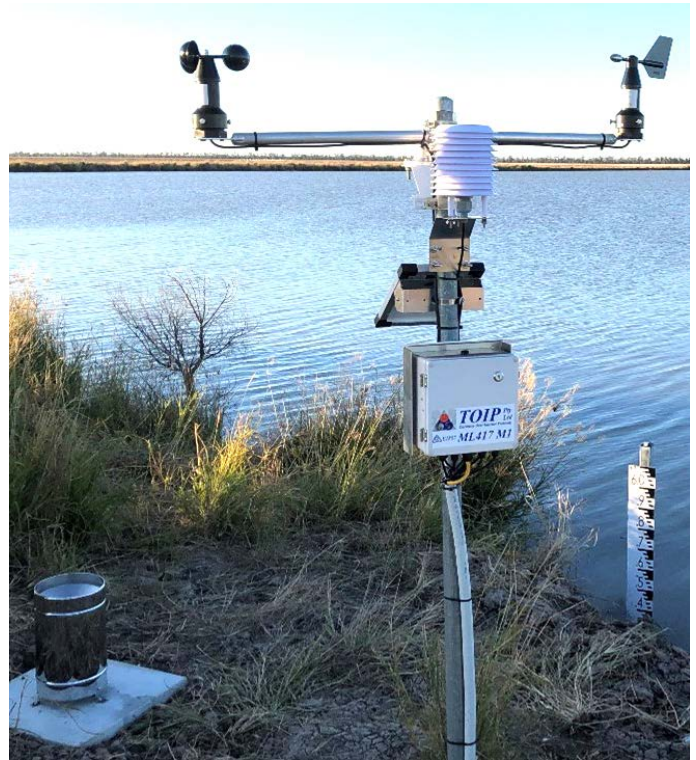
Figure 4. A storage water level, evaporation and seepage monitoring station. A small float in the upper right marks the position of the pressure transducer, which is pulled out to and back from its resting place using ropes in conduit and a pulley.
