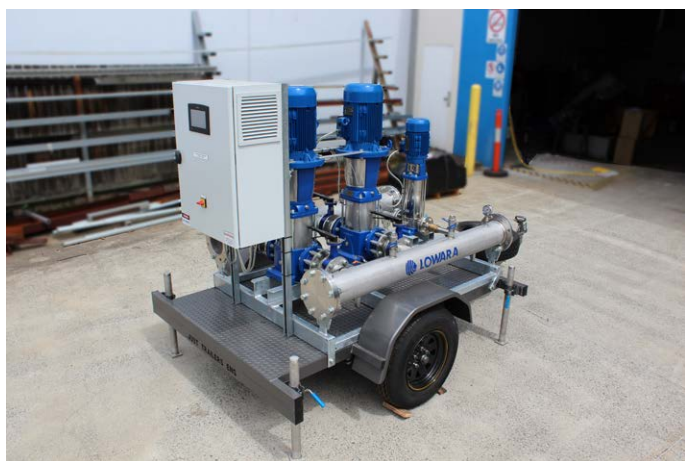
The pumps and control panel are mounted on a trailer. The control panel is mounted with a quick release three-pin electrical connection so the course staff can easily and safely disconnect the power and move the whole pump unit.
