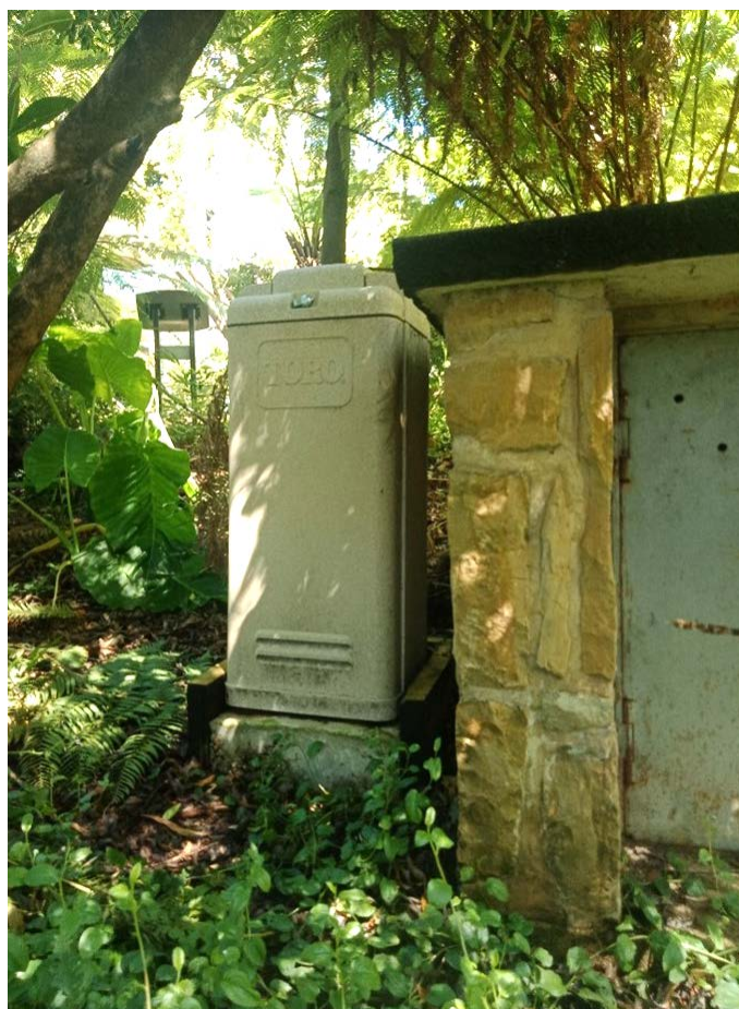
The system relies on smart satellite control in free-standing plastic pedestals throughout the gardens.
